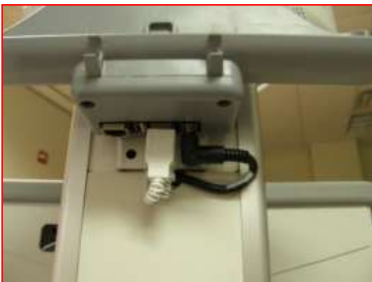
Figure 60. Plugging in Cords to RAM Dock
